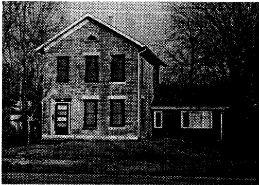
The addition on the right is inappropriate because the height of the addition does not reflect the pattern of the original stone structure.
